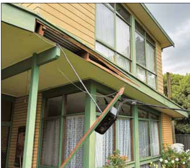
A home's power connection destroyed in the storm. -S
