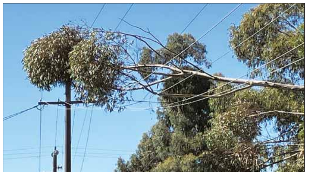
A tree over powerlines. -S
