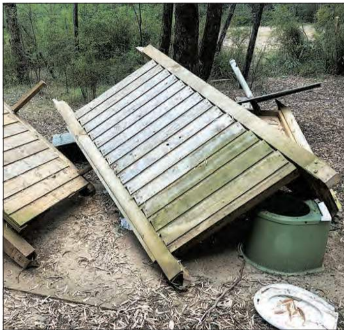
The damaged toilets at the Taponga camping area. -S
