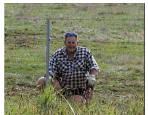
There were plenty of fences needing repairs. -AR
