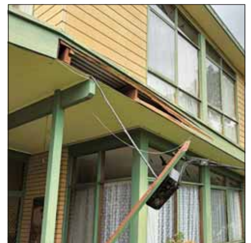
A home's power connection destroyed in the storm. -S
