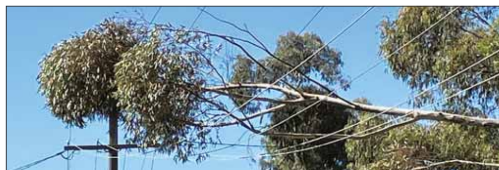
A tree over powerlines. -S
