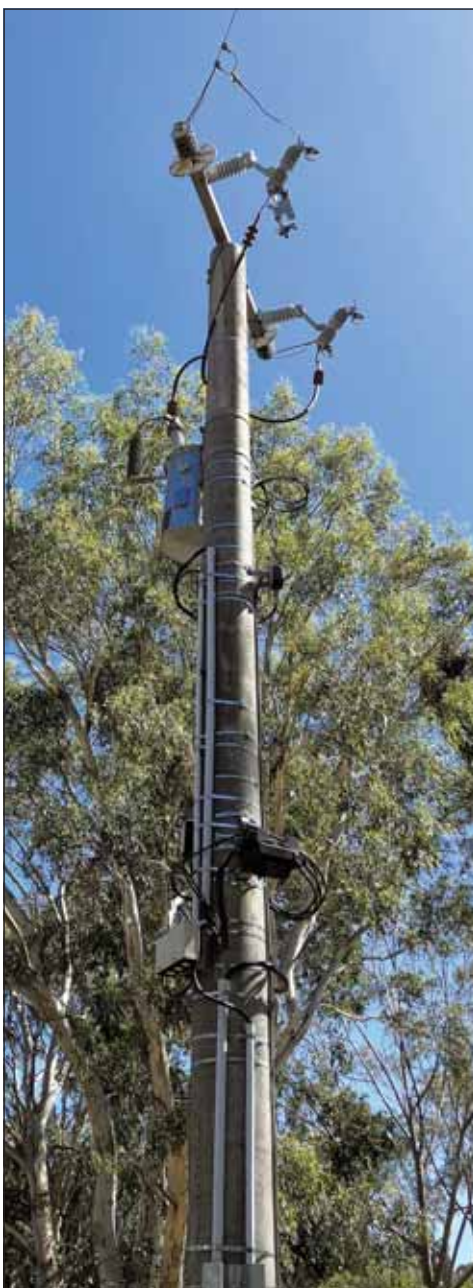
A broken powerline on Halls Flat Road caused the power outage in the immediate area, including Alexandra Secondary College, to last longer than the rest of Alexandra. -S
