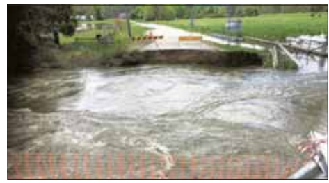
Breakaway Bridge was destroyed in the October 2022 flood event. This image is from shortly after the event. -S
