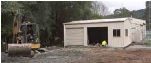
The area around the new workshop getting prepared for paving. - Buxton Fire Brigade
